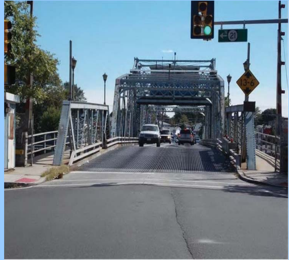
Substandard Vertical Clearance
